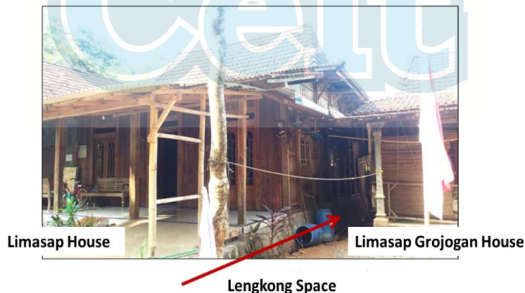
Figure 2: The Lengkong space between the Omah Limasap and Omah Limasap Grojogan (Setiohastorahmanto, 2023)
